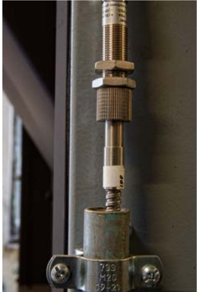
The receiver of the light barrier, connected to a fiber optic protected with a metal sheath, is installed in an area of the furnace whose ambient temperatures are unproblematic for the electronics. (Image: ipf electronic)
