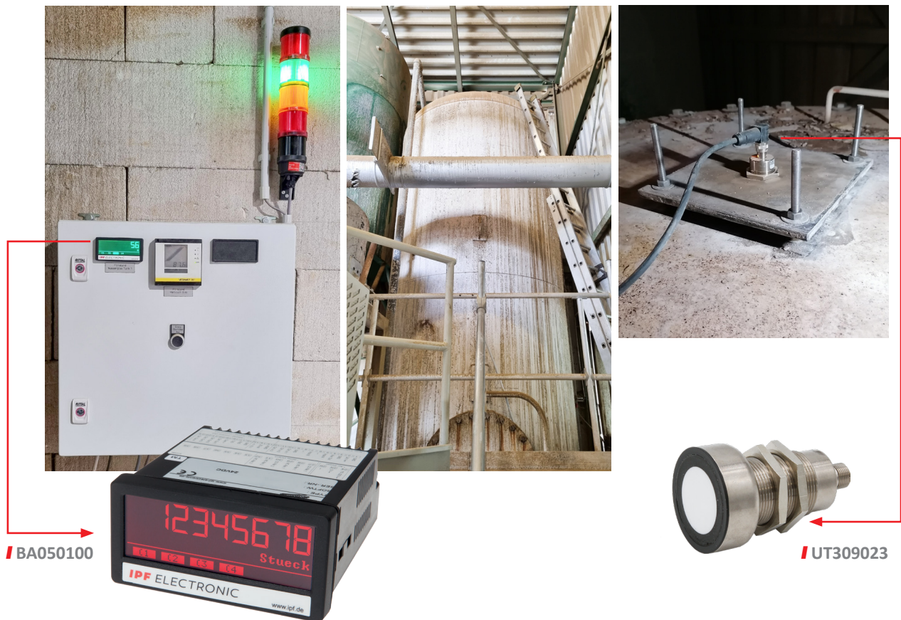
The ultrasonic diffuse-reflection sensor was mounted in the lid area of a silo container (right). The measuring transducer (left) is located in a switching cabinet, near the silo (center).
