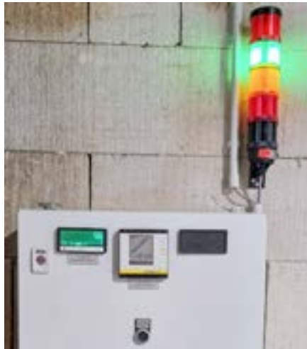
Fig. 30: The display of the BA050100 shows the switching operations of the signal lamps in parallel by corresponding color changes.
