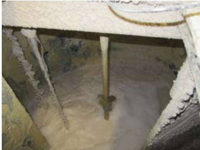
Fig. 34: View into the lime milk tank. To the left of the mixer, the rod probe can be seen, on which only little lime deposits even after longer operation.
