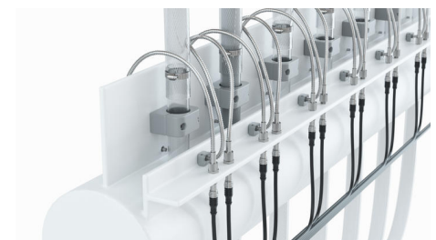
A total of 312 metal-clad fiber optic light guides had to be installed on the glass tubes at the return of the KTL, which were attached to the individual transmitters and receivers.
