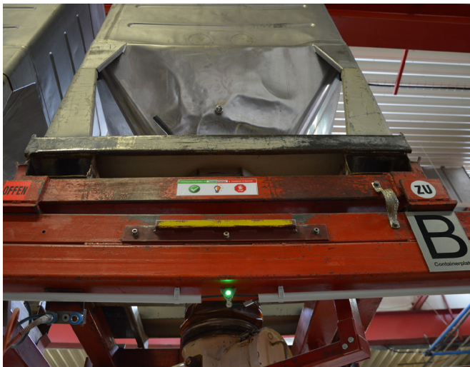
A simple, compact and effective solution: the LED bicolor lights are located below the raw material containers. A green light signals to the forklift truck driver which raw material container needs replacing.
