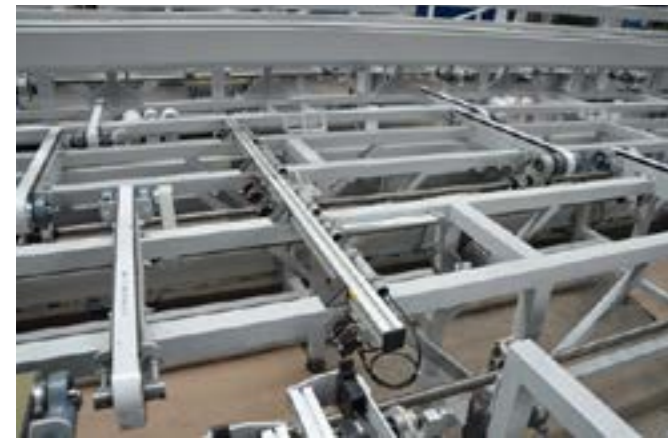
A total of 25 OT430370 optical sensors are used in all areas of the automation solution in which the workpieces are buffered or clocked up.
