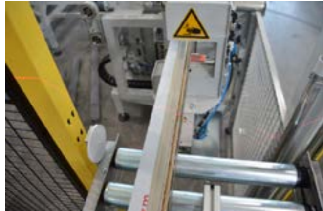
The examination of the profile types takes place on a roller conveyor. There, the pre-fabricated window profiles in another machine are automatically transferred to the system.
