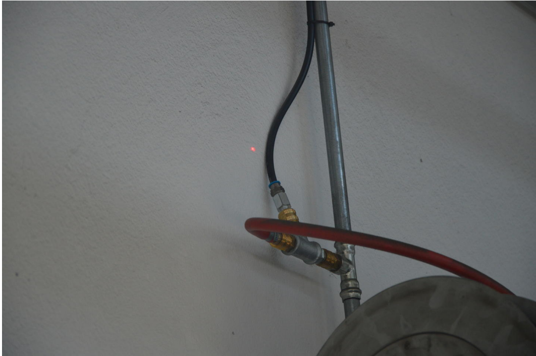
Testing a compressed air line for leaks. The leak detector is equipped via laser distance measurement, which makes it easier to locate the possible leak. In addition, the time-of-flight measurement in combination with the intensity of the ultrasonic signal received by the device can be used to precisely quantify compressed air losses.
