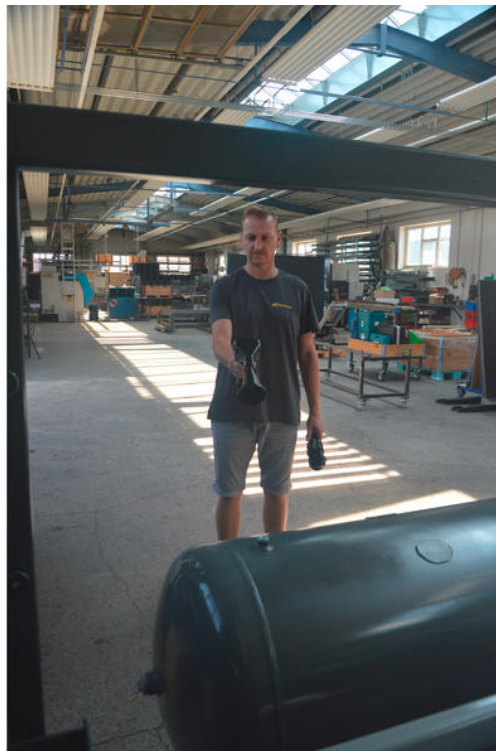
Design engineer Wolfgang Zorn checks the vacuum vessel of the membrane press for leaks using the acoustic funnel of the leak detector.
