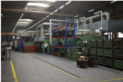
Department with high nitrogen requirements: Kettenwulf's in-house hardening shop.
