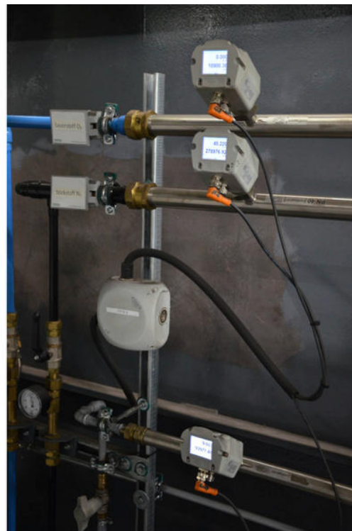
Consumption measurements on a laser cutting system at Kettenwulf: the SY92E297 (above) for the measurement of oxygen, the SY92E296 (center) (reference medium nitrogen) and the SL910020 (bottom) for compressed air.
