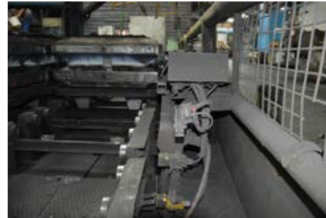
The optical sensors are connected to the system's PLC in order to confirm the casting containers' position within the cooling section via the positional query and, on the other hand, to coordinate the transport of the containers.
