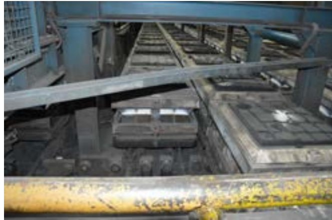
The cooling section runs over a total of 6 lanes, on which the casting containers are transported and positioned in the run-out.
