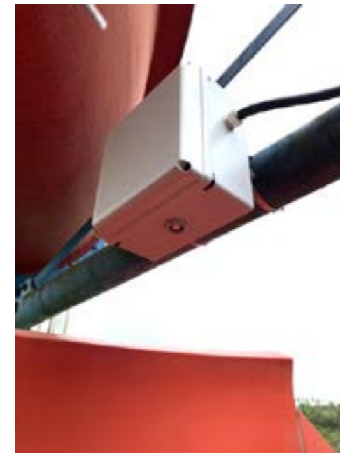
The ultrasonic sensor was mounted above the chute and was then difficult to reach. However, since the analog signal (4...20mA) could be evaluated directly in the control system, the sensor's operating range could be set very conveniently without having to constantly enter the chute for this purpose. (Photo: Martinrea Bergneustadt GmbH)
