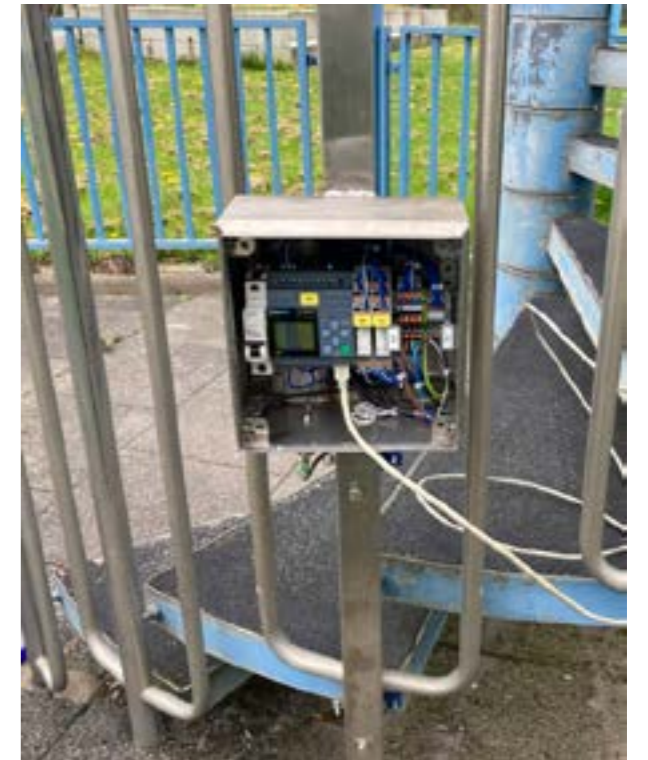
Signal evaluation and further processing of the two sensors is handled by a Siemens Logo connected to the RGB LED signal lamp, with Julian Hooge also handling the complete wiring here. (Photo: Martinrea Bergneustadt GmbH)
