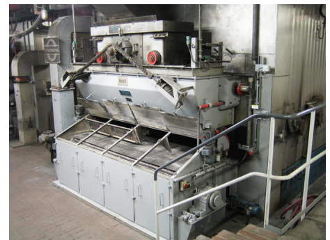
The feed hopper for the fuel is located directly in front of the boiler (in the background) via the traveling grate.
