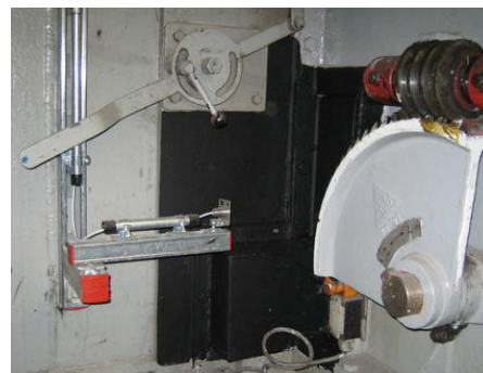
As different temperatures are generated on each side of the feed hopper, an infrared sensor was installed on each side of the hopper (here on the left) for monitoring purposes.
