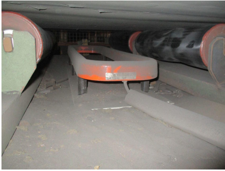
The detector coil under the conveyor belt is mounted with PVC columns on an aluminum base plate that shields against electromagnetic interference from the substructure. This concept also ensures a very stable installation.
