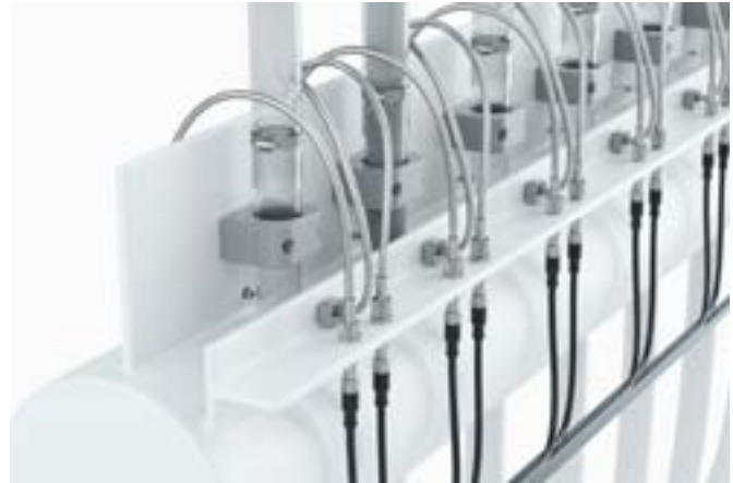
A total of 312 glass fiber optics encased in metal had to be installed on the glass tubes on the return flow of the CDC cooling system and fitted onto the individual transmitters and receivers.
