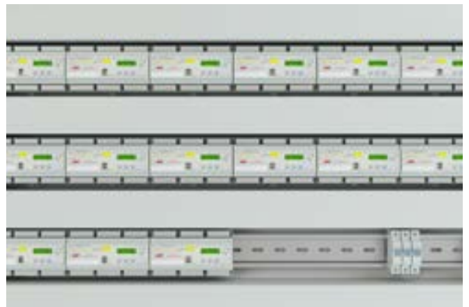
The pluggable transmitter and receiver elements were connected via conventional sensor lines to 20 evaluation units located in a separate switching cabinet. The amplifiers allow the transmitting power to be adjusted both manually and automatically (for a high level of soiling compensation).
