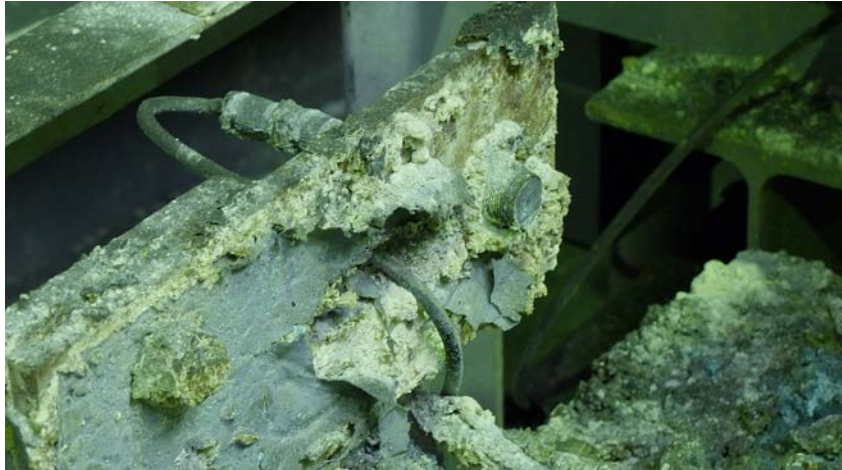
Hardly recognizable: The acidic pickling process is extremely the laser light barriers in the buffer zones.
