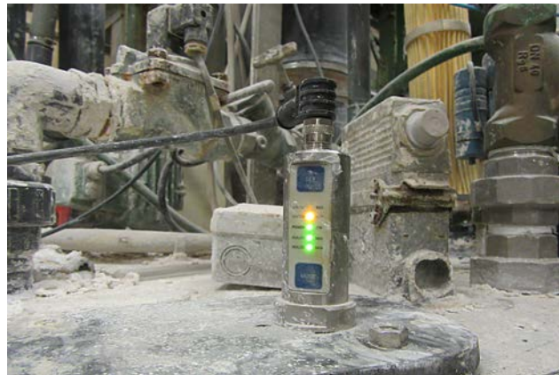
The housing and the connection of the capacitive level sensor are made of stainless steel. The limescale deposits are also clearly visible on the container of the preparation unit.
