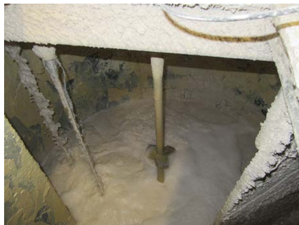
In the container, the lime is mixed with water to form milk of lime. To the left of the mixer is the PTFE rod probe, on which only a small amount of lime deposits even after prolonged operation.
