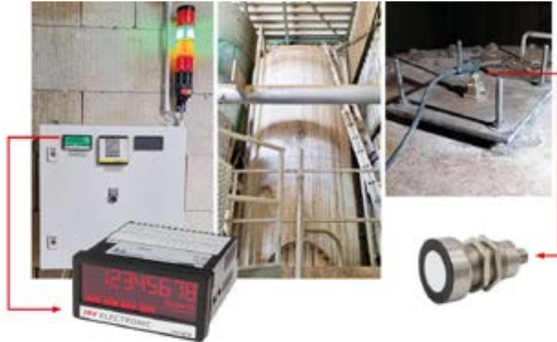
In this application, the ultrasonic probe was mounted in the lid area of a silo container (right). The measuring transducer (left) is located in a switching cabinet near the silo (center).
